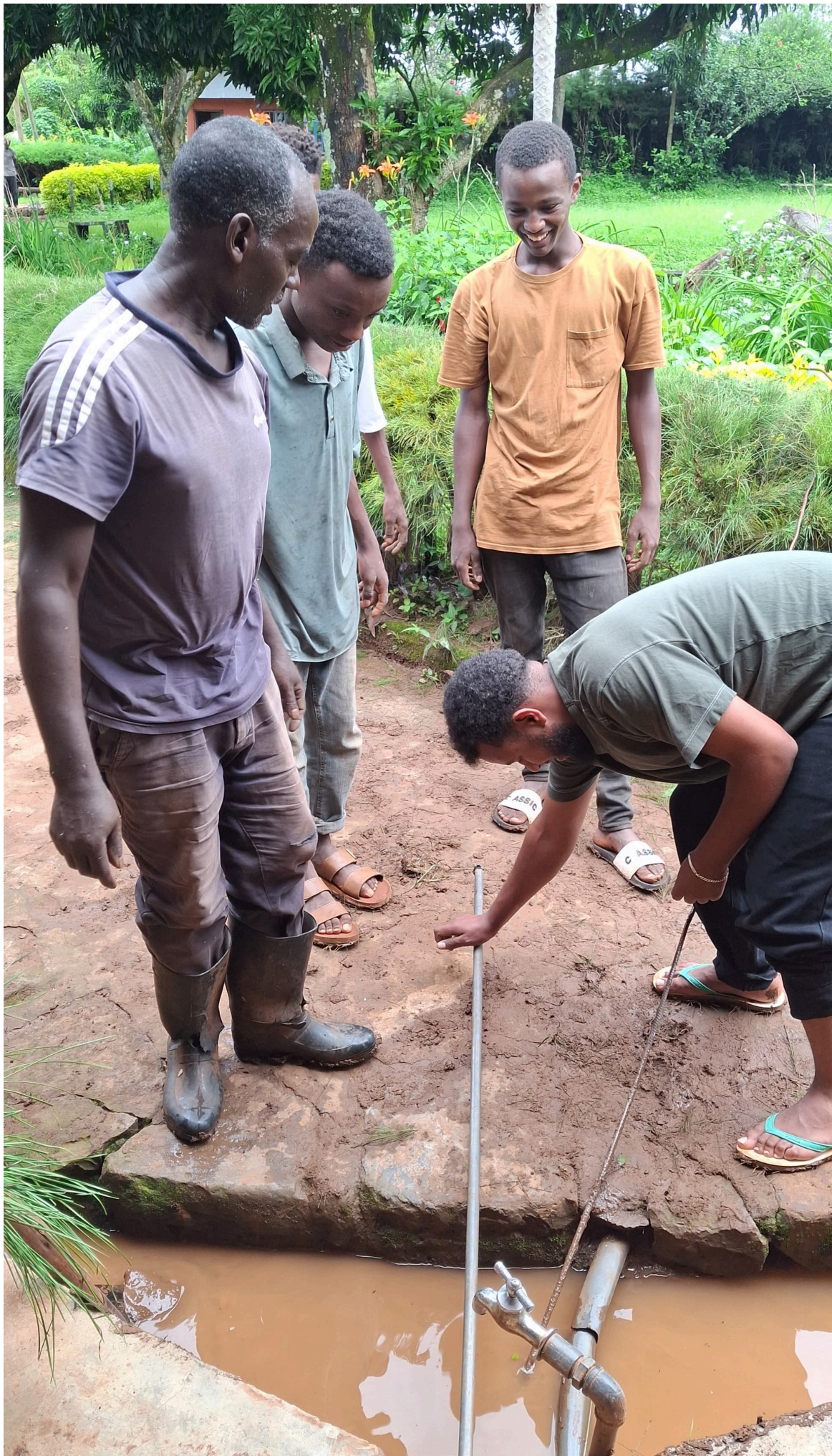
Work being done to unblock draining pipe to reduce water pools and mosquito breeding. Sami (right) is working with little more than a metal pile and rope.
